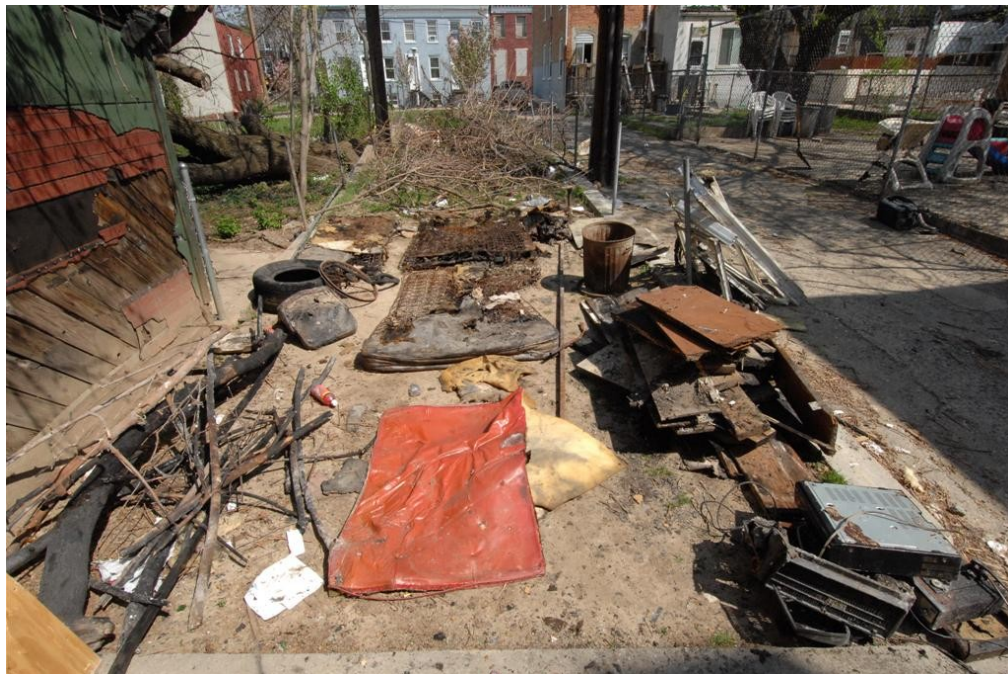
Debris on concrete pad after removal from rear room.
