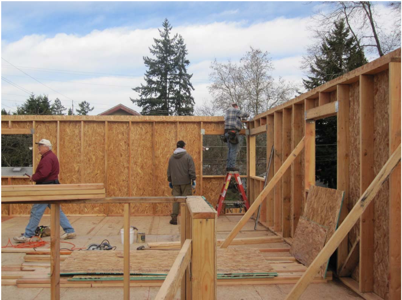
This is one of the latest pictures from the site; they almost have all the exterior walls of the 2nd story built! Good job guys! From left: Family Support Committee member Doug Bartlett, Event Committee member Andrew Schafer, and volunteer Thomas Venzke.
